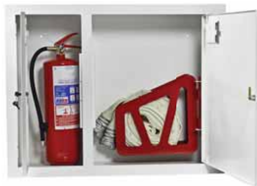
Fire hose reel cabinets
